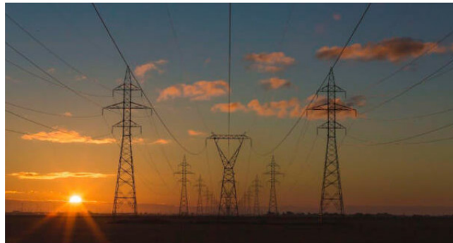
Electricity pylons at sunrise OR sunset, unidentified location. Original public domain image from Wikimedia Commons
